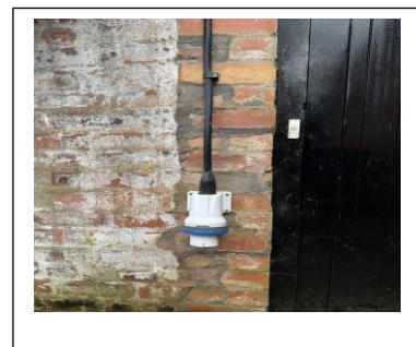
External Generator Hook up
