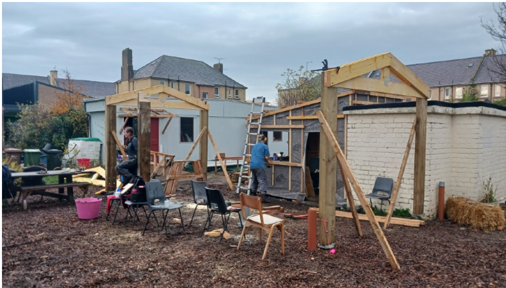
Construction of a new permanent shelter, for outdoor community meals and other activities
