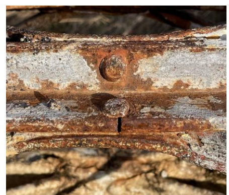
Sprung rivet can be seen on the left, and a fracture by the rivet on the right.
